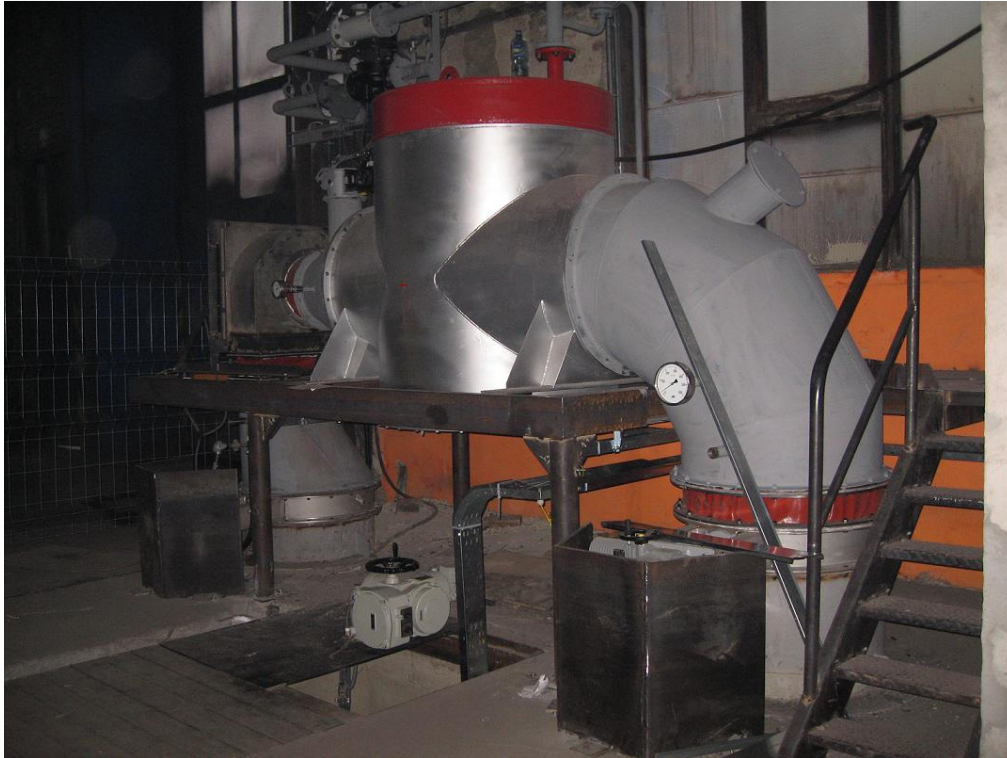
Image 2 Econotherm GW unit in operation
